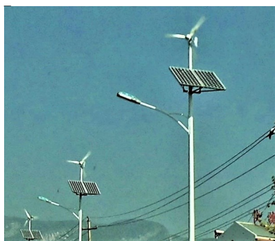
Combined wind and solar power to light the road near Pingyao, Shanxi province
